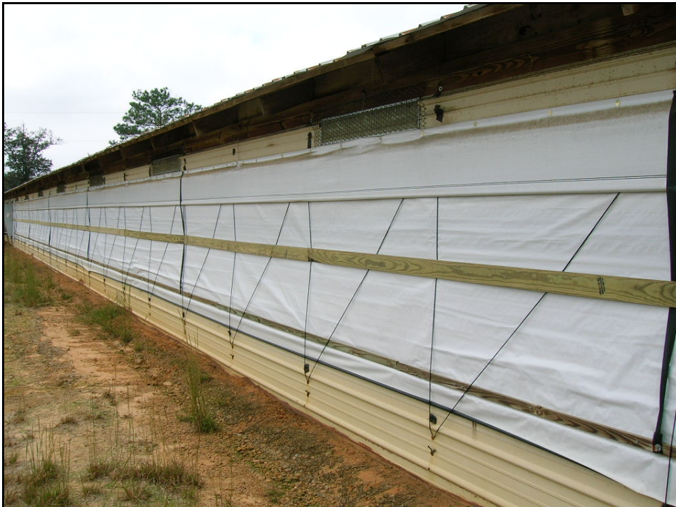
Nailed Down Curtain – October 2005
